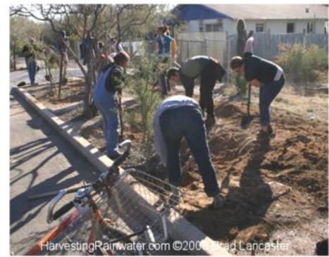
Volunteers converting a roadside to a rainwater catchment rain garden in Tucson, AZ.
